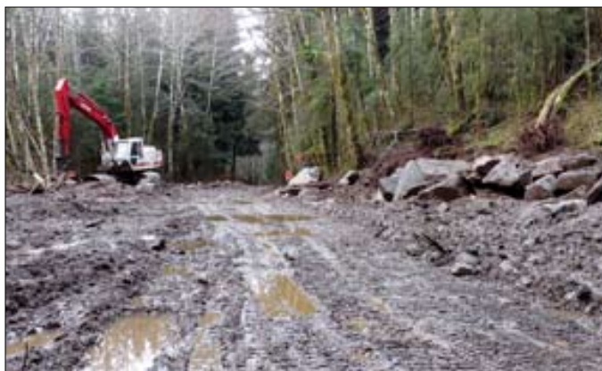
A contractor well-acquainted with SSRAA infrastructure re-buried the pipeline and provided better protection against bad weather to come.
