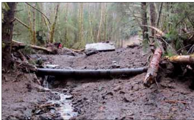
The pipeline carrying the critical water supply for Neets Bay Hatchery was exposed and vulnerable after a violent, wind-driven rainstorm.
