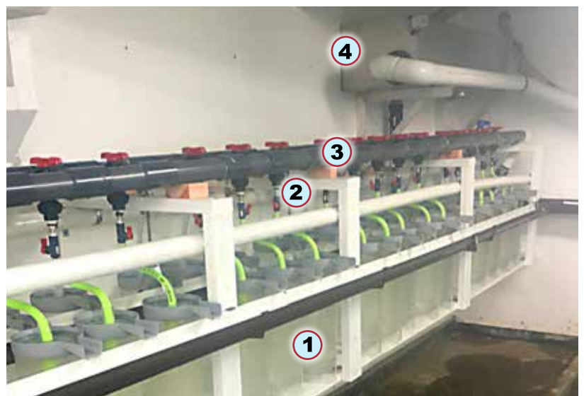
The experimental incubator array at Deer Mountain Hatchery: 1) hatching jars; 2) valves; 3) water supply pipes; and 4) head box.
